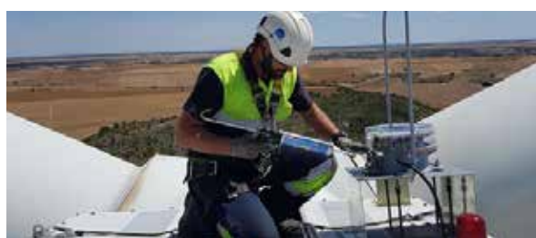
EÓLICA WIND POWER
